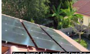
Source: HopSol Africa, residential installation
