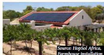
Source: HopSol Africa, pv roof installation in the central of Namibia
